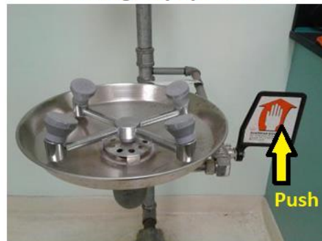
Emergency Eye Wash
